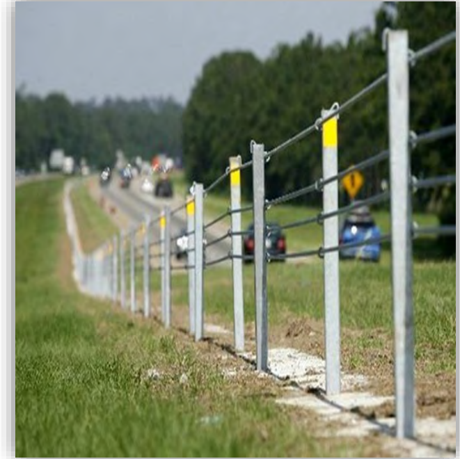
High Tension Cable Median Barrier
