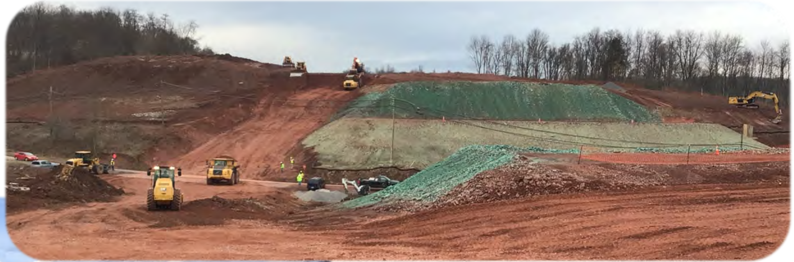
Embankments for Bridge Abutments and Temporary Haul Road Crossing at Grangers Road
