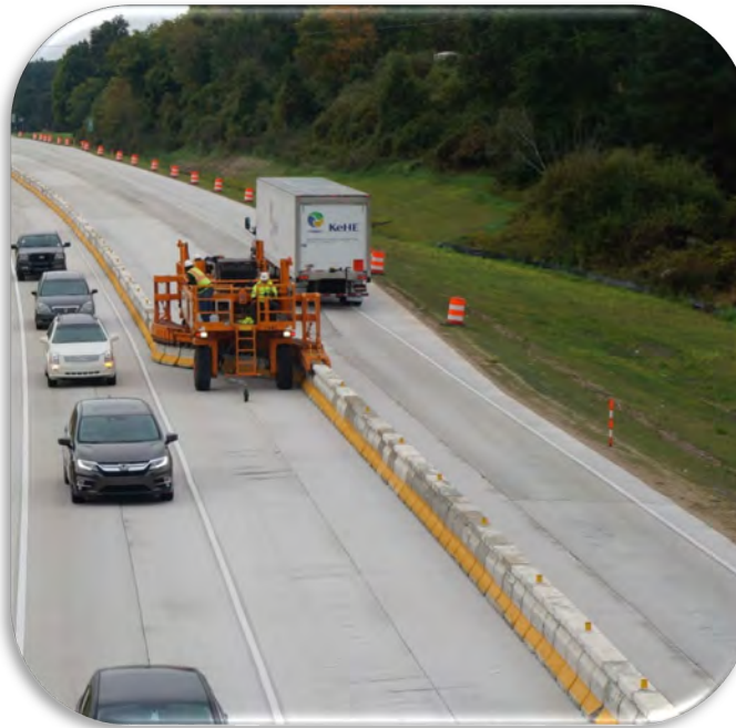
Moveable Median Barrier
