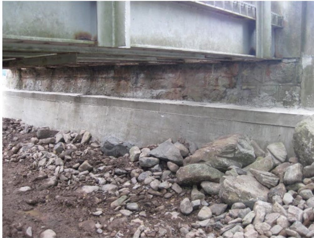
Near abutment. Note the abutment has been underpinned and a reinforced concrete apron has been installed.
